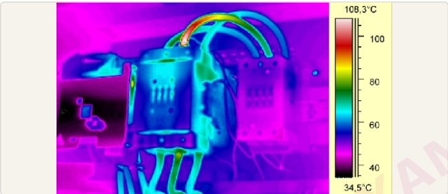
Sönke Krüll, „Elektroschuetz”, Wikimedia Commons, CC BY 3.0 – unmodified · Contactor cable termination: ≈ 108 °C while neighbouring conductors stay at 35–60 °C.
