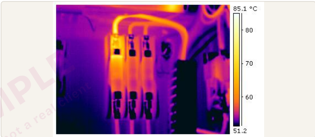
Hofflashhome, „Electrical fault”, Wikimedia Commons, CC BY-SA 3.0 – unmodified · One phase is hotter than the other two – the textbook case for comparing with similar components.
